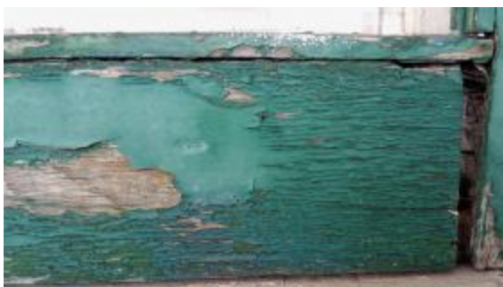
The "alligatoring" pattern of the peeling paint is a tell-tale sign of lead paint.
