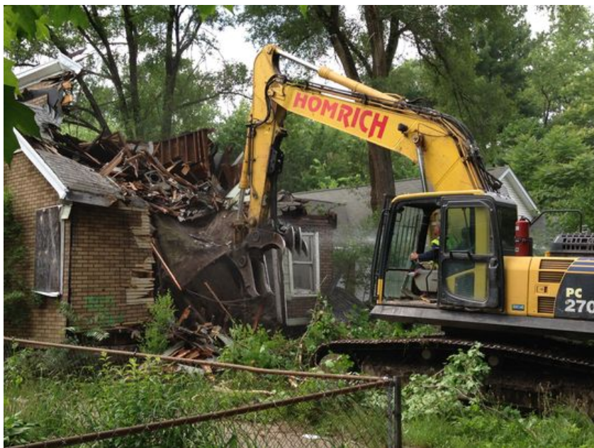
A contracted demolition crew from Detroit-based Homrich demolishes a house on Dolphin Street, as part of the city's blighted house demolition program (Photo: Keith Matheny)
